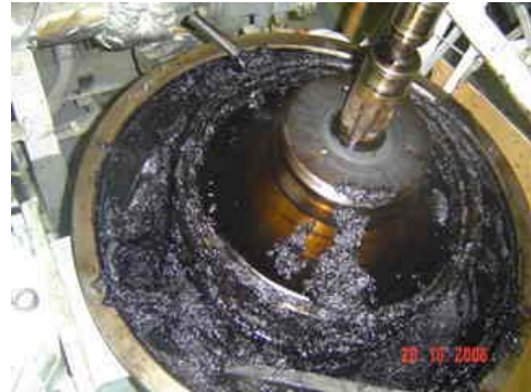
Fuel deterioration from long-term storage leads to sludge-laden purifiers like that shown here. PRI-RS application to the fuel prevents fuel degradation. With treatment, the fuel will remain fresh for months, even years at a time.
